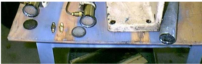
A close up of the pumps and meter units.
